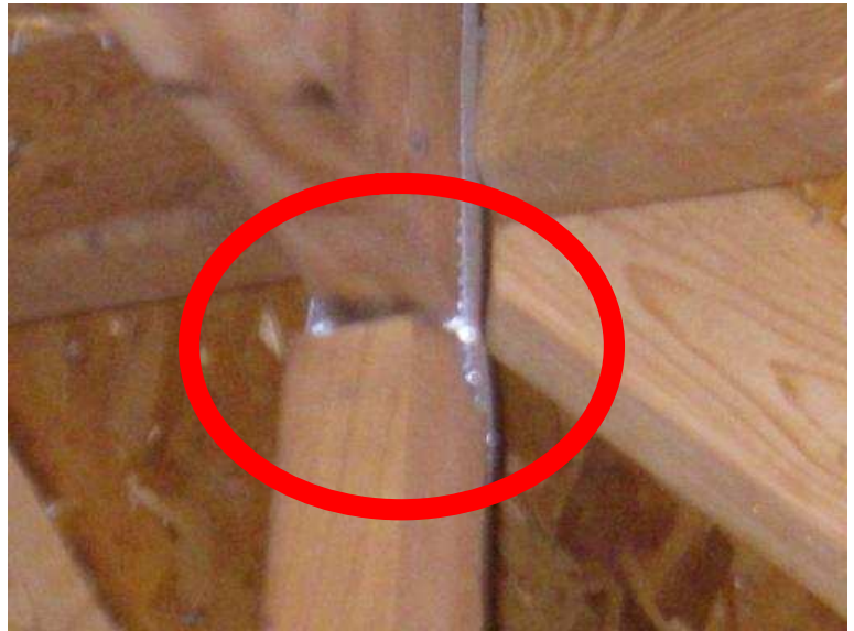
Main Attic Area -, Loose/damaged truss plate on the roof truss (1st truss to the right if the right end hip intersection)
