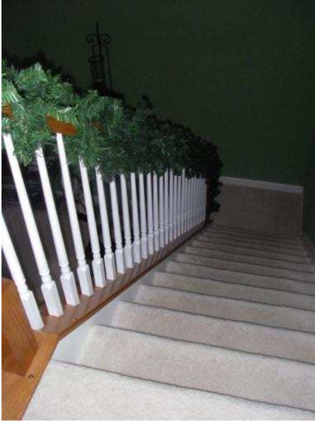
Loose handrails right side stairs
