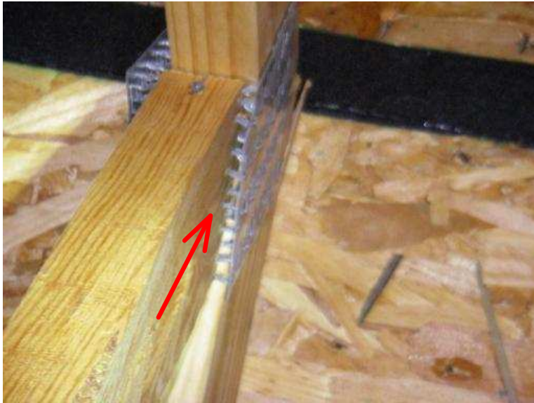
Loose truss plates on roof truss
