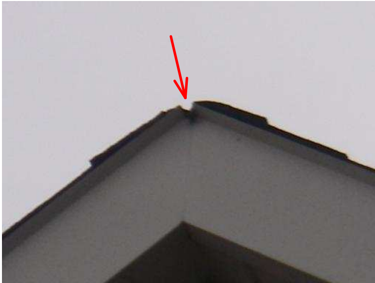
Ridge cap shingles are split on the front gable ends
