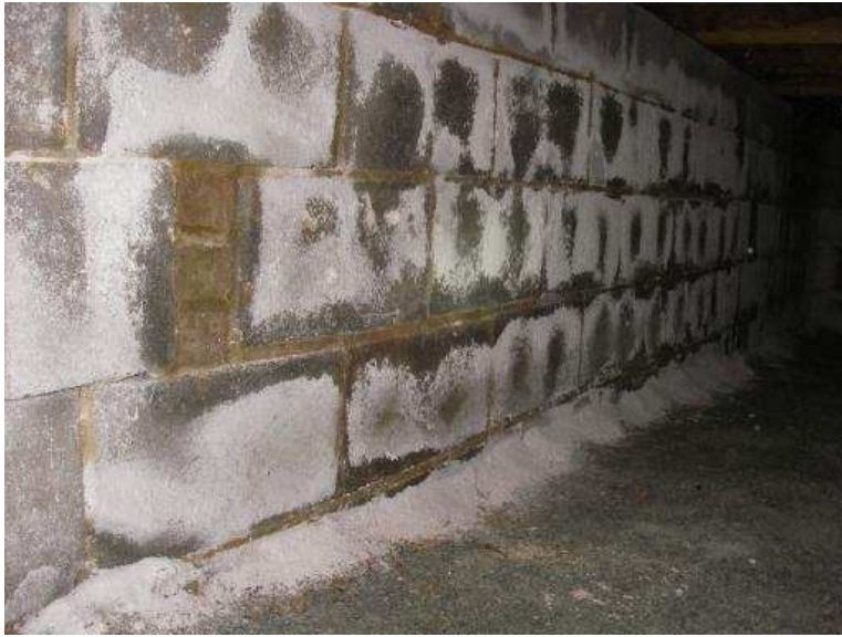
Efflorescence was observed on the foundation walls
