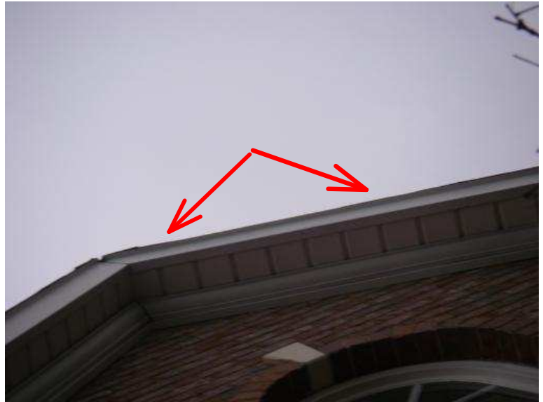
Insufficient shingle overhang along the right side of the garage front gable
