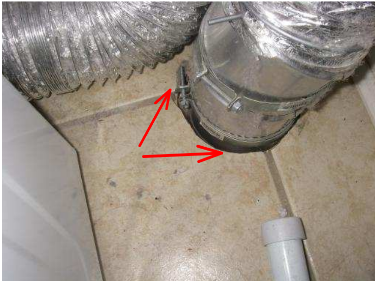
Properly seal penetrations in the flooring in: laundry room
