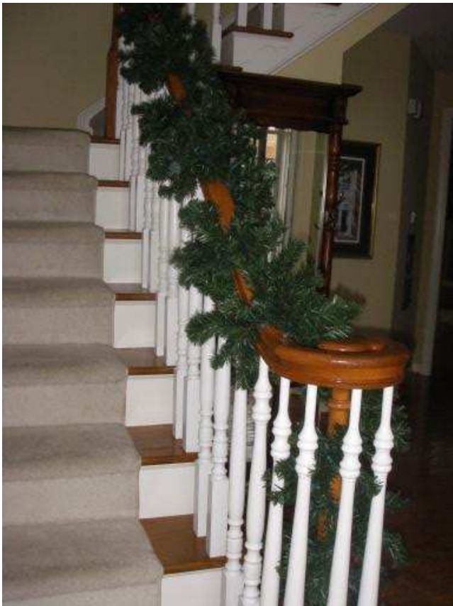
Loose handrails along stairs
