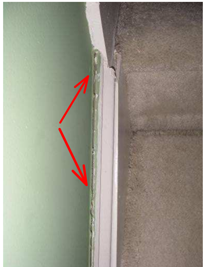
Loose trim at the bottom landing (right side stairs)
