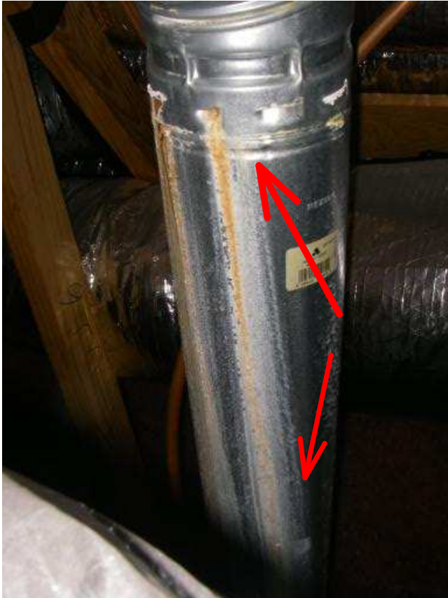
Rust is present along the furnace exhaust stack (in attic)
