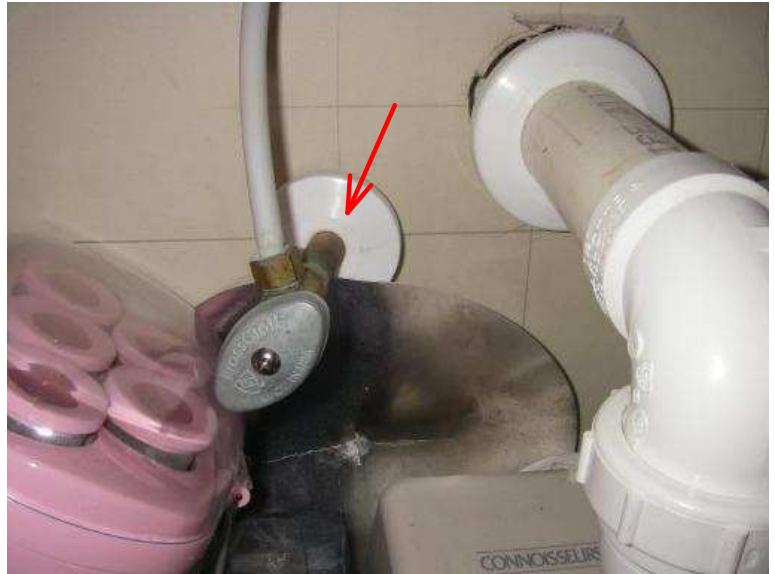
The hot water supply line is not properly secured in place inside the wall cavity - master bathroom
