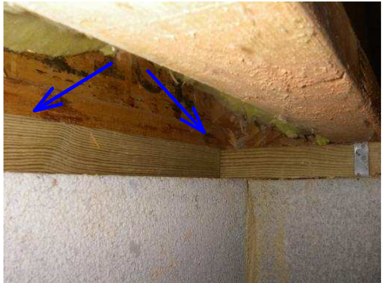
Anchor straps /bolts are not visible within 12 inches of some of the corners in the crawl space
