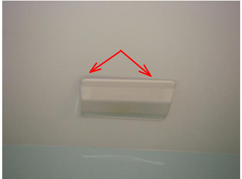
Loose fan at ceiling level in 2nd floor bath
