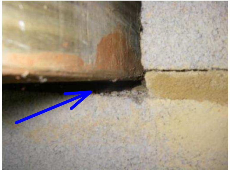
Piers not in contact with the right end of the interior girder
