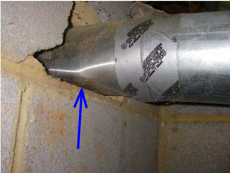
The dryer vent is crimped in the crawl space
