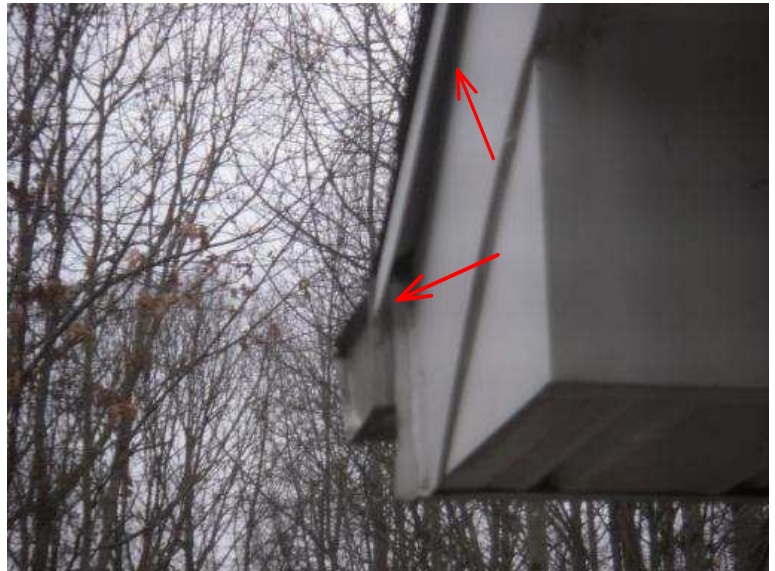
Loose fascia rear wall
