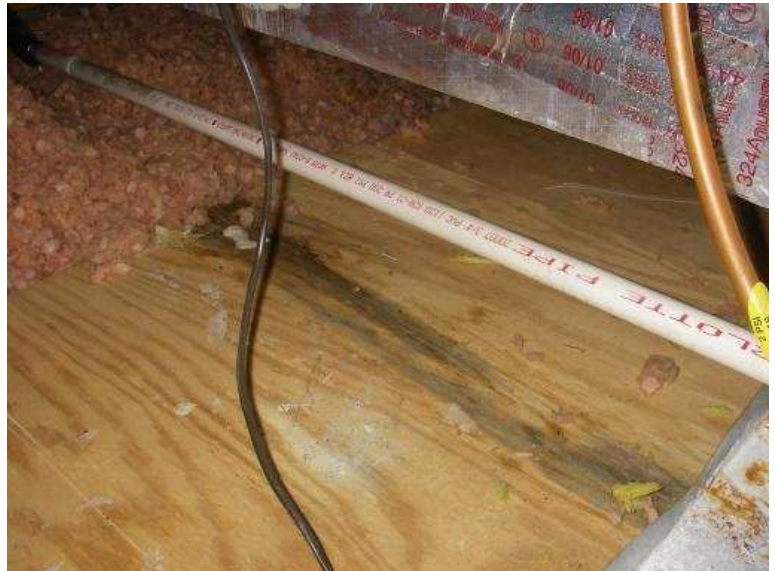
Evidence suggests the condensate drain pipes are dripping in the attic
