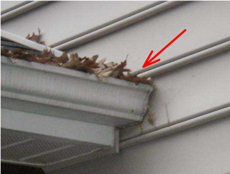
There is no visible kick-out flashing at the bottom junctions of the lower roof slopes and house
