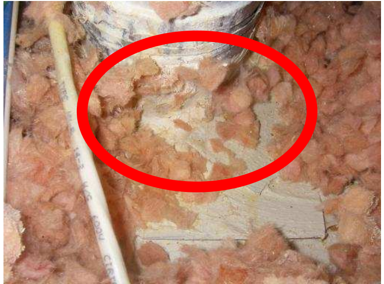
The ceiling is wet at the bottom of the furnace exhaust stack in the attic area
