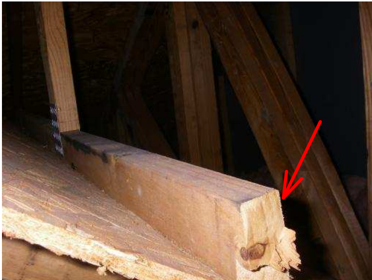
Front Gable (Attic) - Roof truss bottom chord has been cut-in-two.
