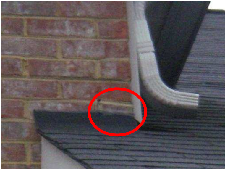
Loose brick at the right front corner of the wall-to-roof area and flashing
