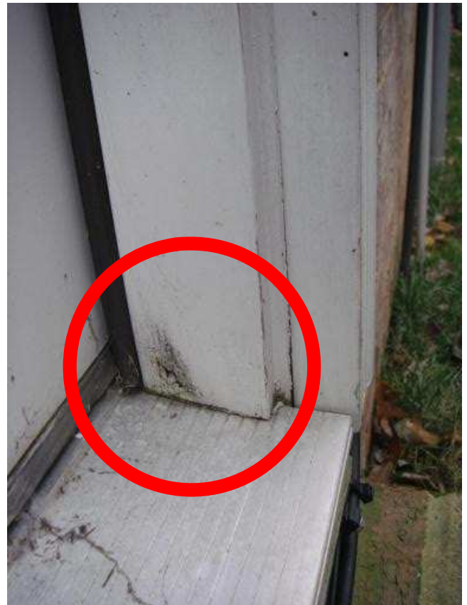
Damaged trim /frame at the right side garage service door
