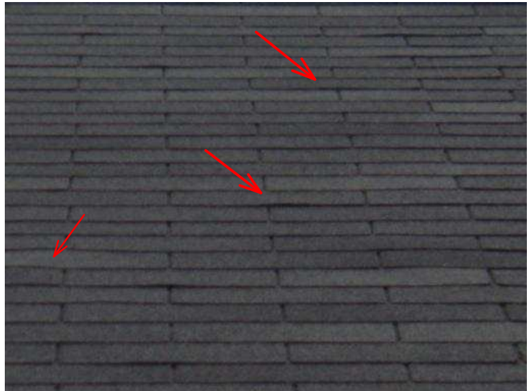
Nail back-out in shingles
