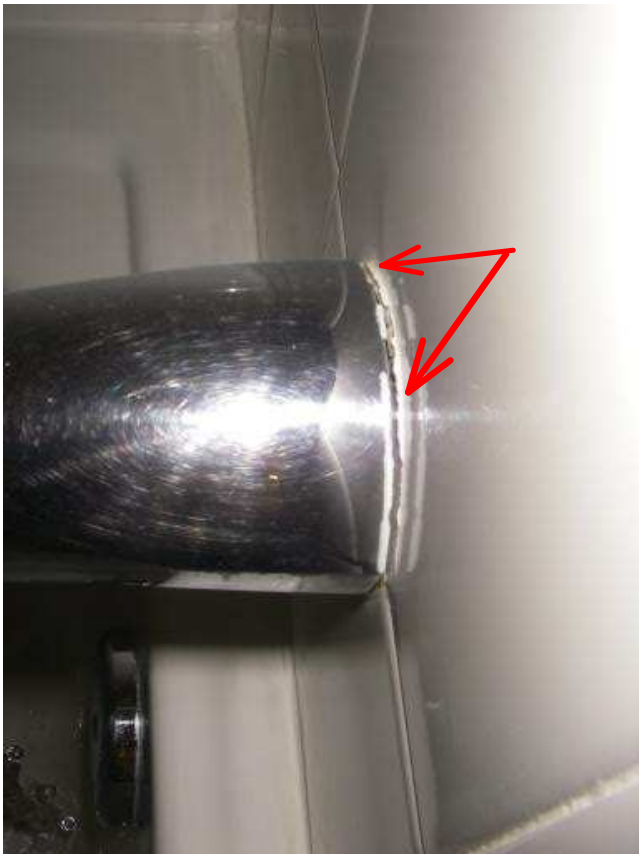
Tub fixture needs caulking
