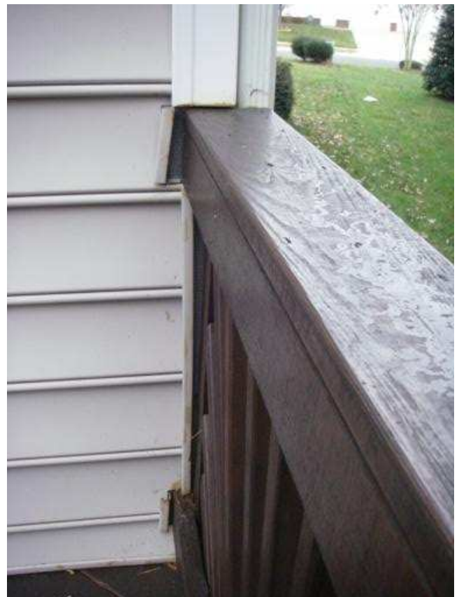
Deck rails are loose and need securing.
