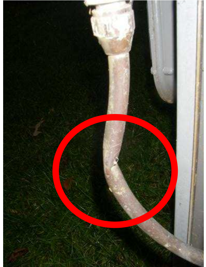
Gas Meter - The copper gas pipe is severely crimped
