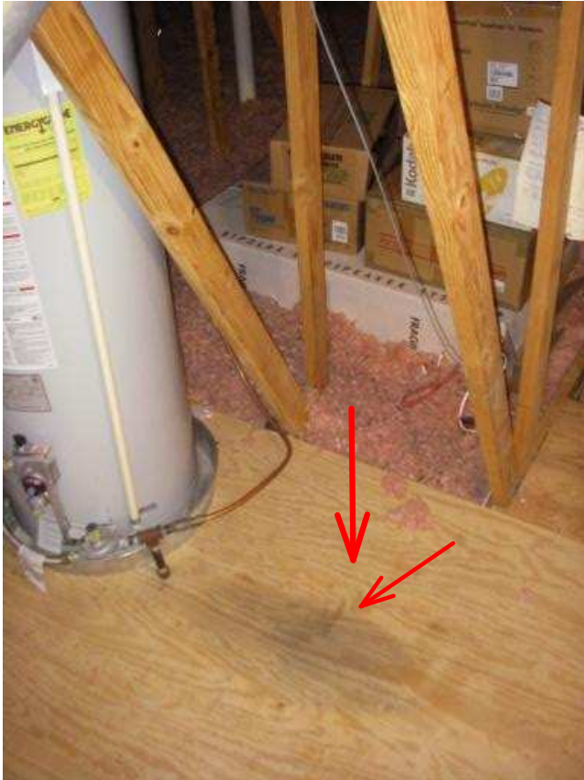
Evidence of prior moisture intrusion below the furnace exhaust stack in the attic.
