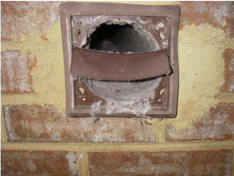
The exterior dryer vent cover is damaged
