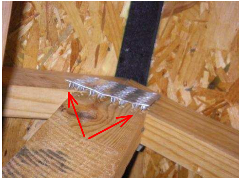
Main Attic Area - Loose/damaged truss plate on the roof truss
