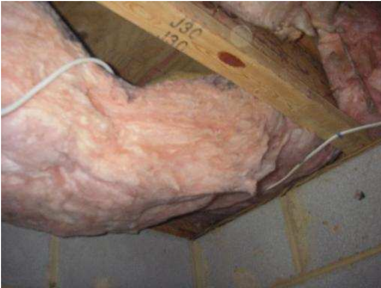
Crawl space insulation is falling down in various locations
