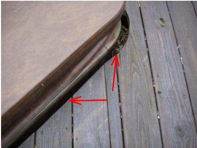
FYI - Gap between the hot tub and deck can and may pose a step through hazard for a small child.
