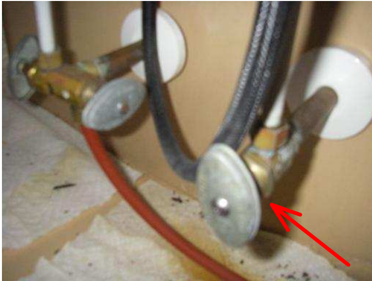
Leak at cold water valve (kitchen sink)
