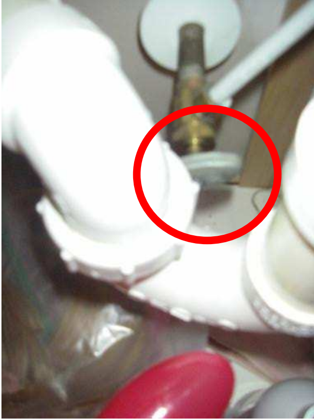
The cold water valve in contact with drain pipe
